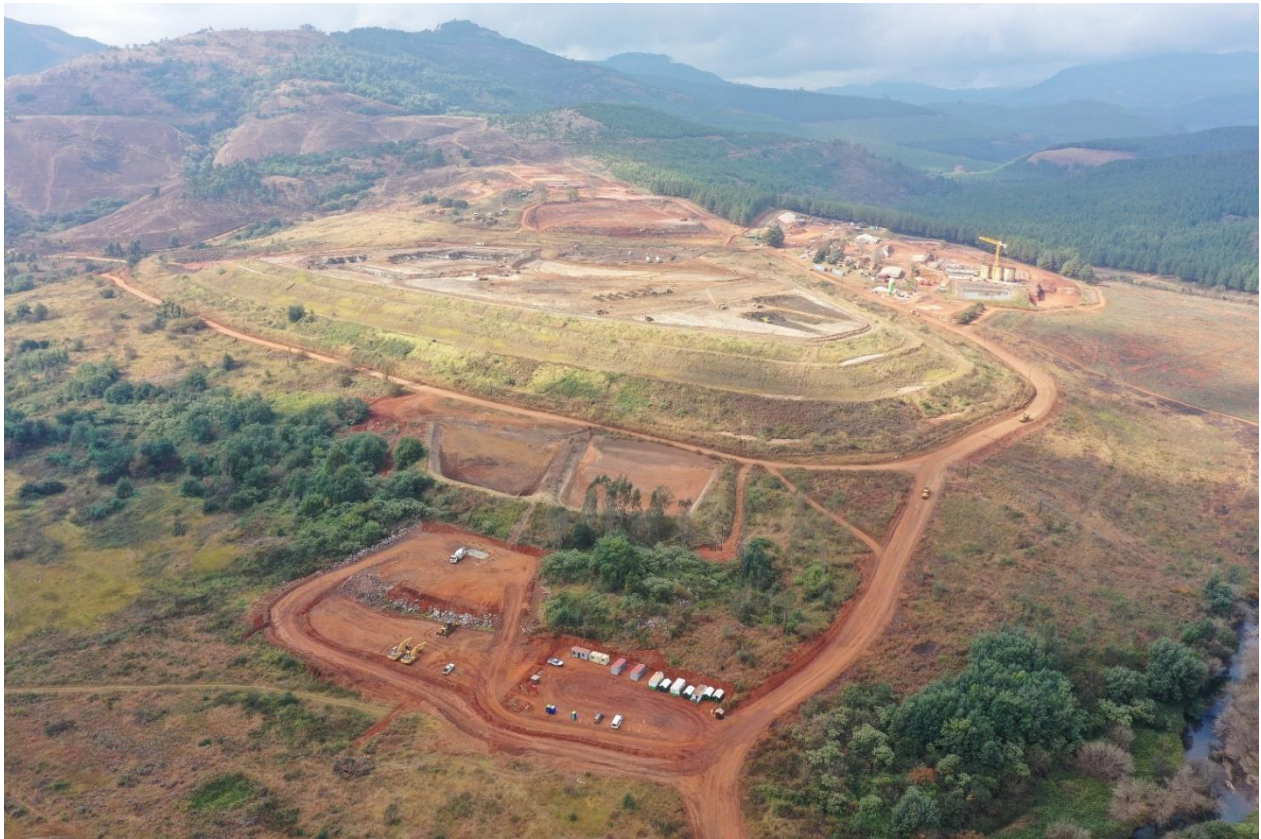
Figure 1: TGME Gold Project aerial view of the TSF (bottom: Laydown area ; middle: TSF; top right: new plant under construction).
