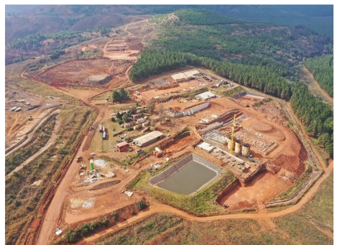
Figure 3: Aerial view of TGME site highlighting plant footprint and integrated construction progress
